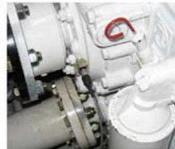
CMCP1100 Vibration Transducer One for each Gear
